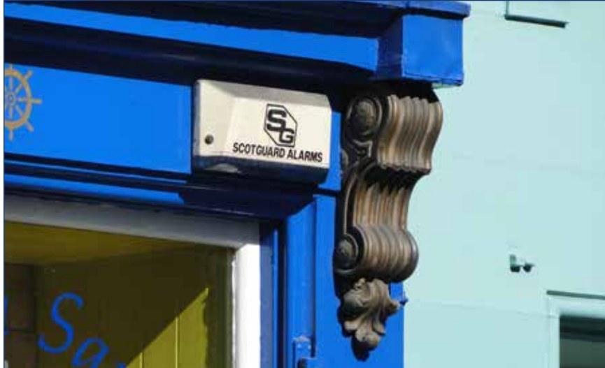
Burglar and fire alarm boxes should be carefully located in as inconspicuous a position as possible. This image illustrates bad practice.
