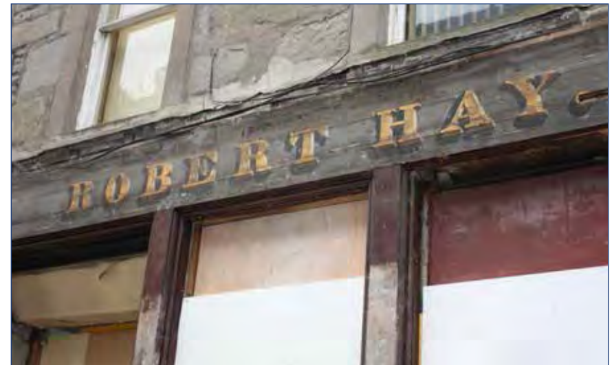
On-site dountaking of modern layers can reveal historic detailing. © Courtesy of Lindsay Lennie, Historic Shopfront Conservation
