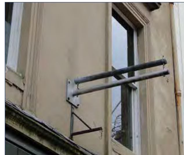
Banners and other large scale advertisement displays including new flagpoles should not be located on the front elevations of buildings located in conservation areas or on listed buildings as they have a detrimental impact on the amenity and appearance of these historic buildings and places.
