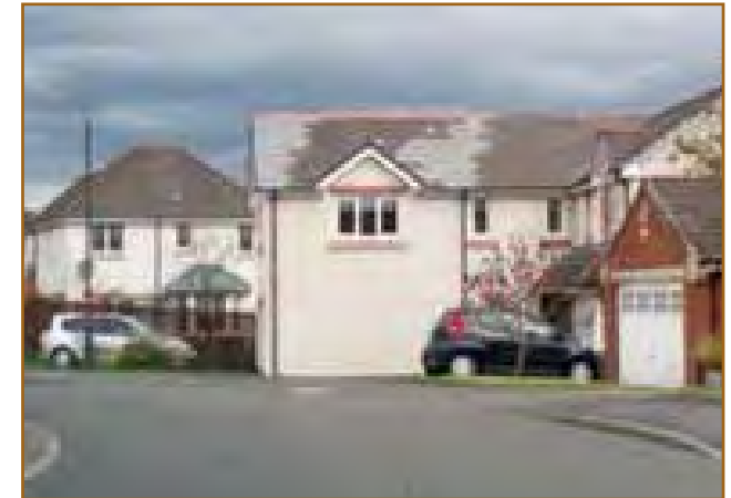
Figure 6b: Poor Use of Materials & Design
