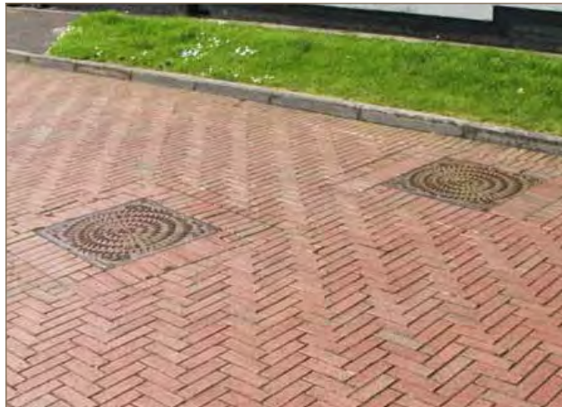
The accommodation of utilities should not affect the layout/design of roads and footways.
