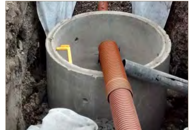
Utilities can be integrated into a service strip at the side of the roadway as a means of easy maintenance.
